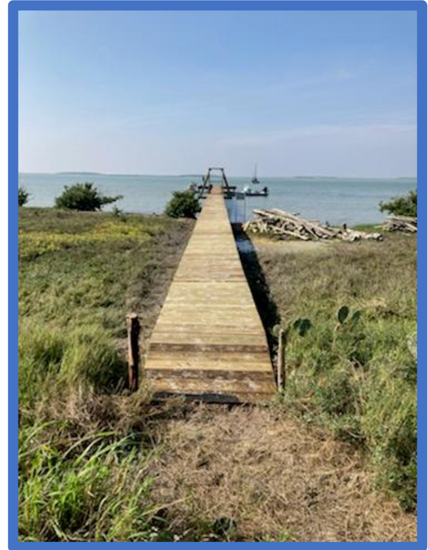
SEP funds from an Audubon Texas project were used to build a new dock for conservation activities at green island, 2022 (SEP No. 2011-52)
