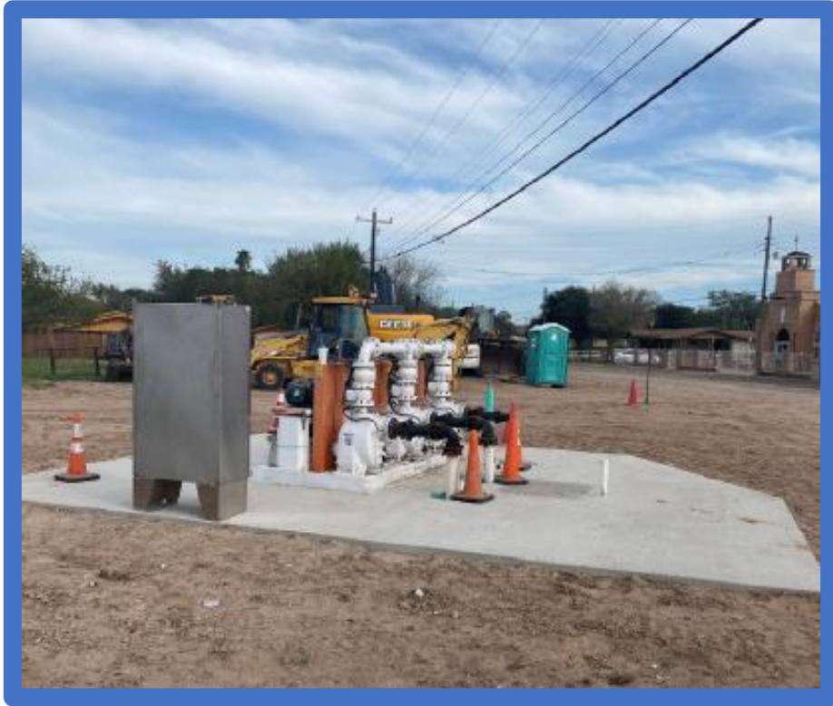
Rio Grande City, Texas installed a new Lift Station with backup pump at their facility, 2019
